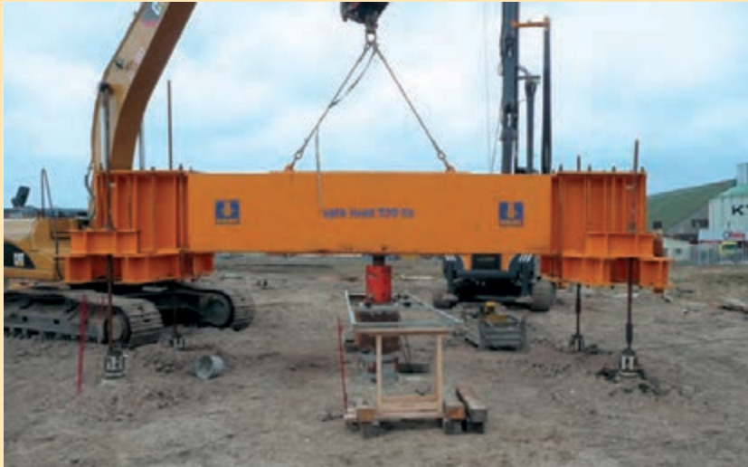
Pile load test reaction beam for a maximum test load of 3200 kN
